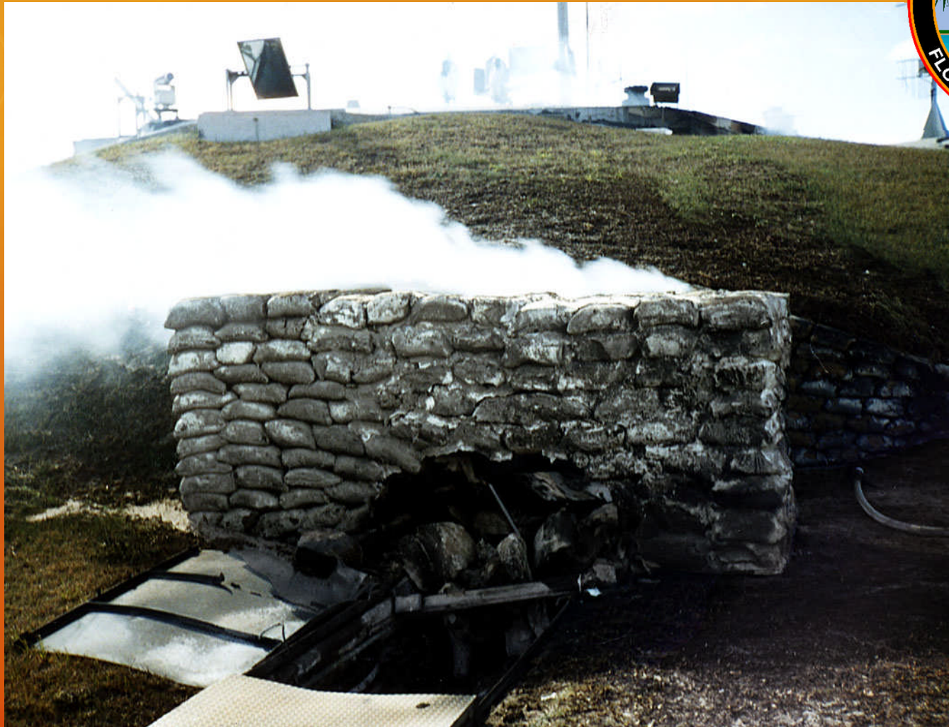
Cable tunnel problem area
